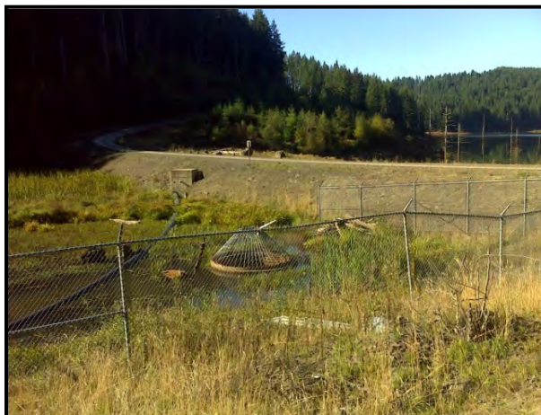
Photo C-6 View of earthen dam and water control structure at the Barney Reservoir Arm 2 mitigation wetland site.
